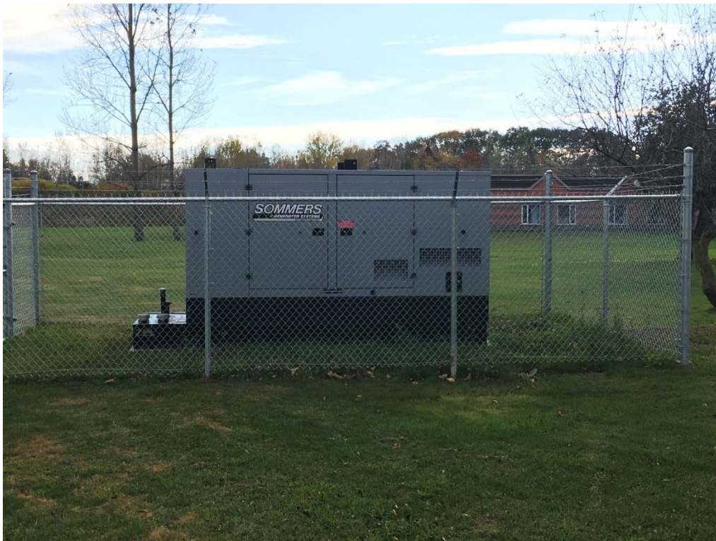
Figure 6. Back-up Generator at the Senior Citizens Complex
