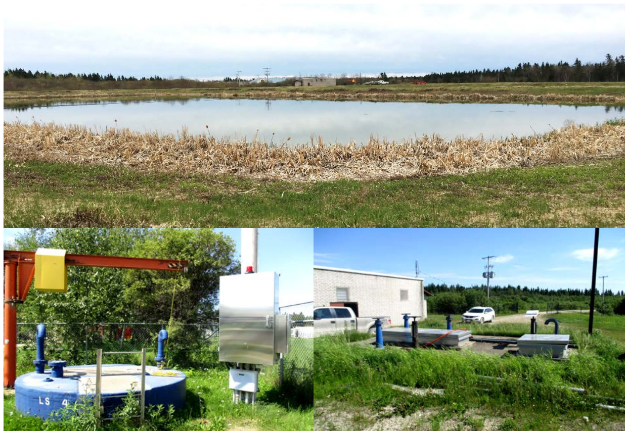
Figure 12: Typical Lift Station, Lagoon Cell, Valve Chamber and Blower Building
