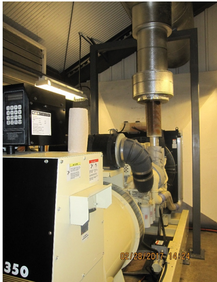
Figure 11: MCA Water Treatment Plant Backup Generator
