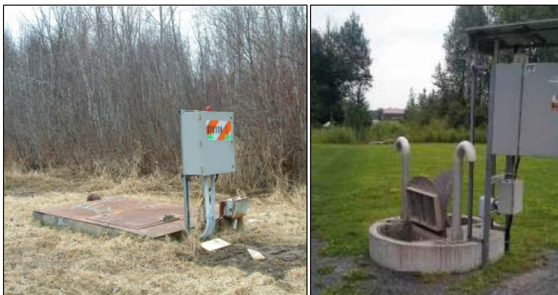
Figure 24: Snye Pump Station #1 (left) and Pump Station #2 (right)
