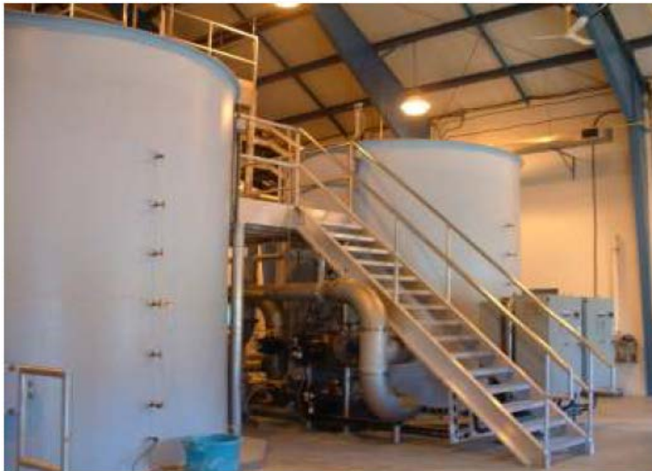
Figure 18: Granular Activated Carbon Tanks at St. Regis WTP
