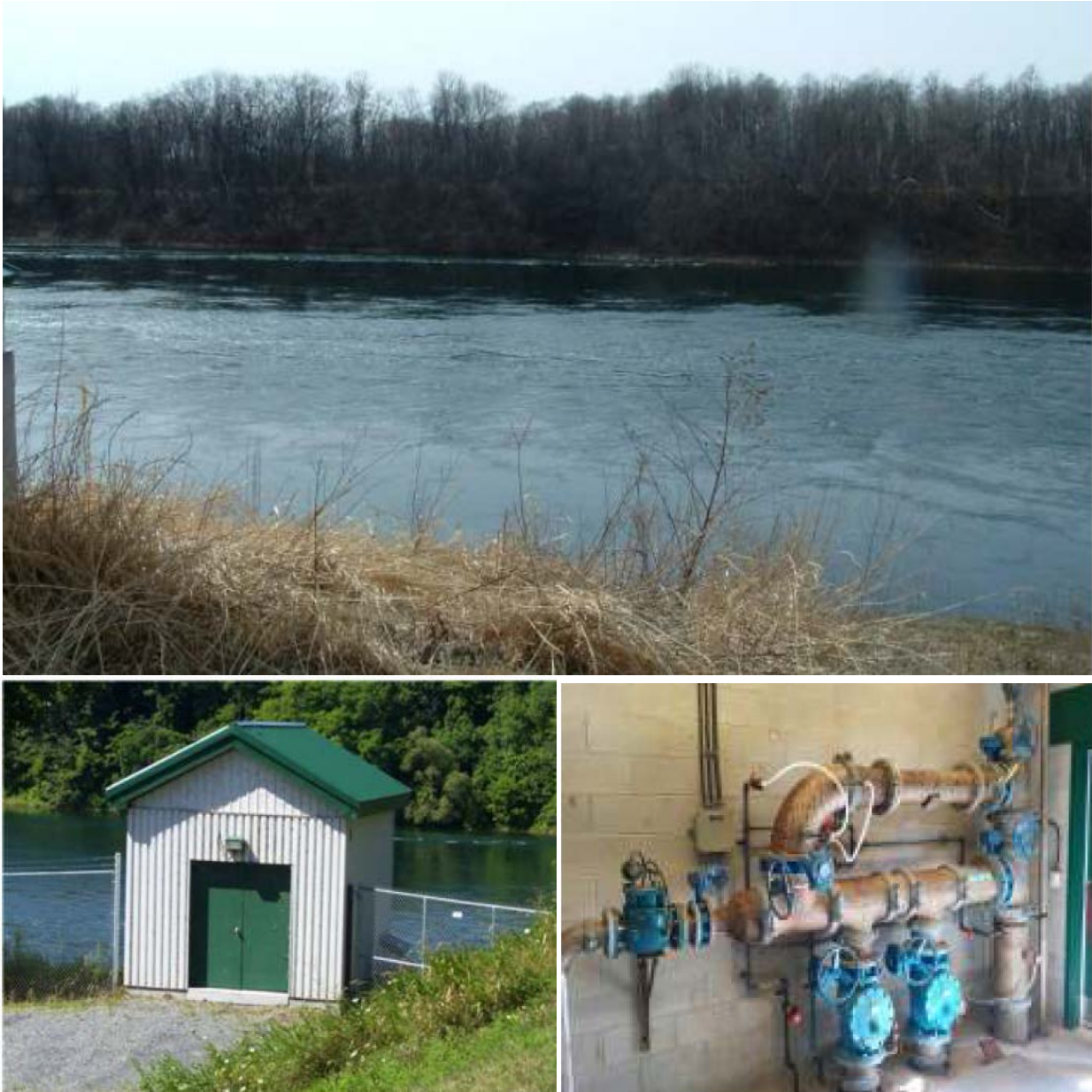
Figure 8: Intake and Low Lift Pump
