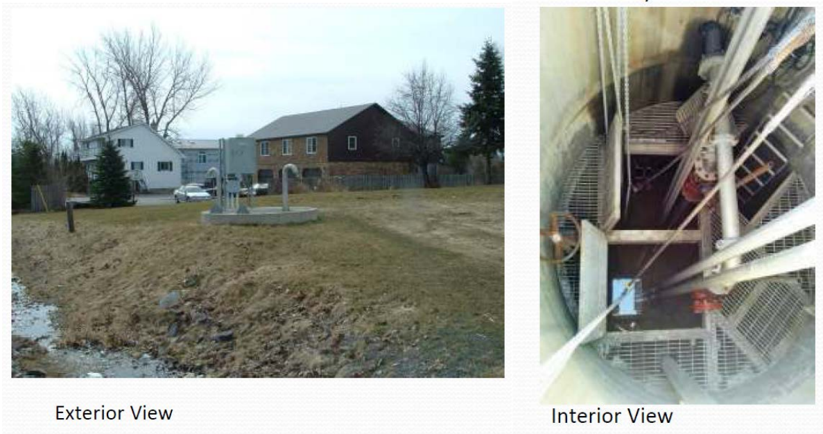
Figure 14: Exterior and Interior Views of the Cornwall Island Administration Pump Station
