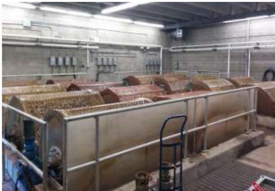
Figure 22: RBC Units at St. Regis WWTP
